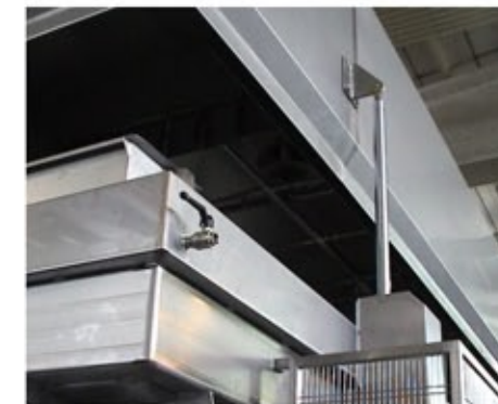
Insulated and sealed (hood) outer envelope, with mechanical lifting system for washing and maintenance operations
