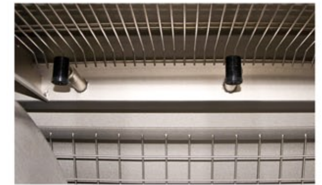
Nozzles for further water sprinkling on the product
