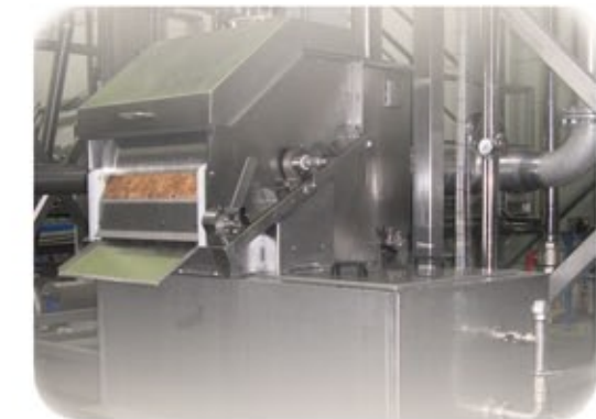
Filtration unit with tank and return pump for the water used by the sprinkling shower system
